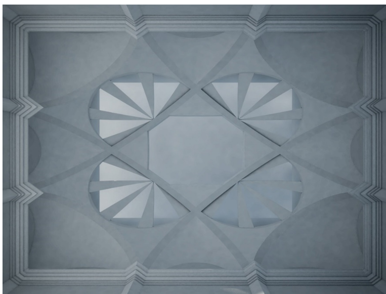
Fig. 6. Perspective view of the digital reconstruction of the vault in the Castle of Racconigi.
