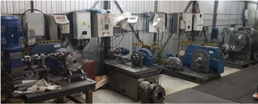
Fig. 10 a Small Innovative Enterprise “Mechanic” (machining site). b Small Innovative Enterprise “Mechanic” (testing site)
