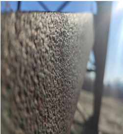
Fig. 1. Pitting corrosion of support elements.
