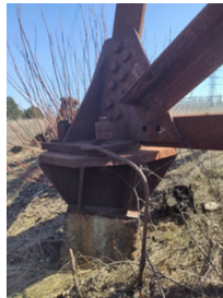
Fig. 2. Traces of deep corrosion of the joints of the support elements.
