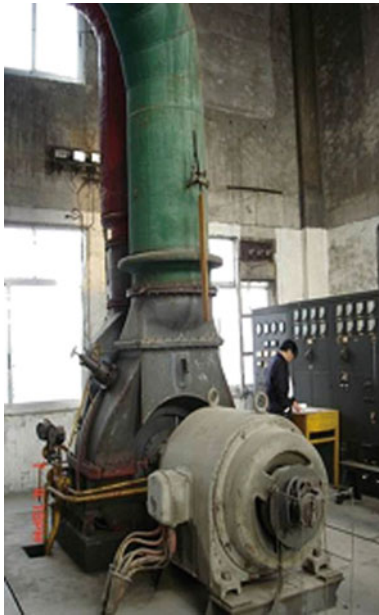
Fig. 5 300 kW geothermal power station in Fengshun, Guangdong. Reproduced with permission from Ref. (Zhu et al. 2015). Copyright @ Elsevier Inc. (2015)
