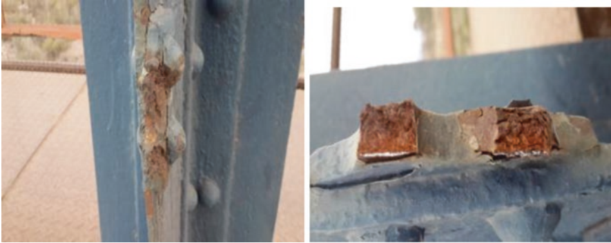
Fig. 12.45 Macroscopic observation of the structure of the bridge, column detail from third section and external corrosive damage
