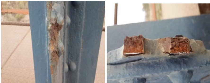
Fig. 12.33 Macroscopic observation of the bridge structure, column detail of the third section and the external corrosive damage produced
