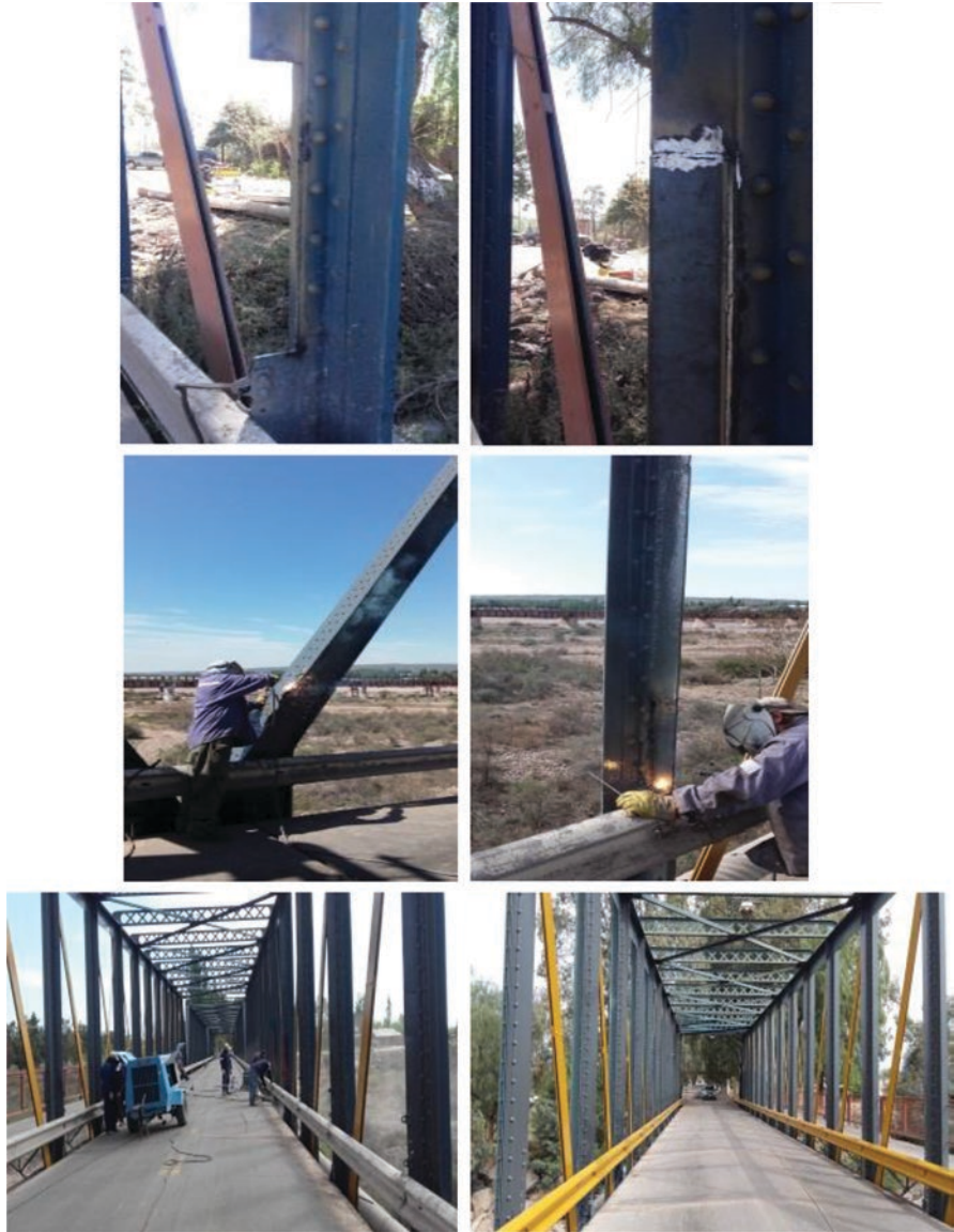
Fig. 12.47 Details of repair work, surface preparation, welding, and painting of the old iron bridge over the Mendoza River
