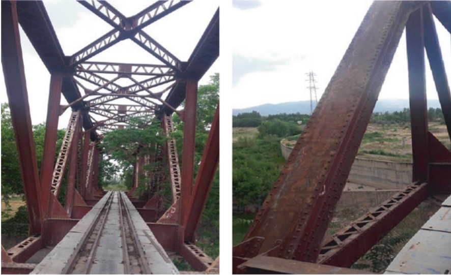
Fig. 7.1 Uniform corrosion in steel structures of FFCC N°2 Railroad, Luján de Cuyo, Mendoza, Argentina
