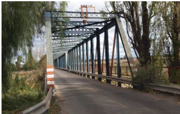
Fig. 12.30 Panoramic view of the iron bridge over the Mendoza River in its North-South direction
