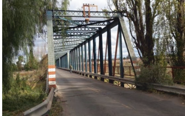
Fig. 12.42 Panoramic view of the Iron Bridge over the Mendoza River in its north-south direction
