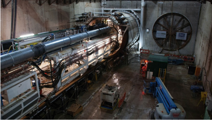
Fig. 1 Example of a complex construction site; Plumstead Tunnel with Tunnel Boring Machine (TBM) on Crossrail Thames Tunnel Project
