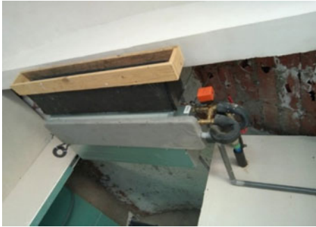
Fig. 5 Fan convector built-in, bungalow of Hammam Righa spa, Algeria
