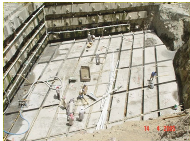
Fig. 1 Execution of GW flow system under tower F following GW model outputs
