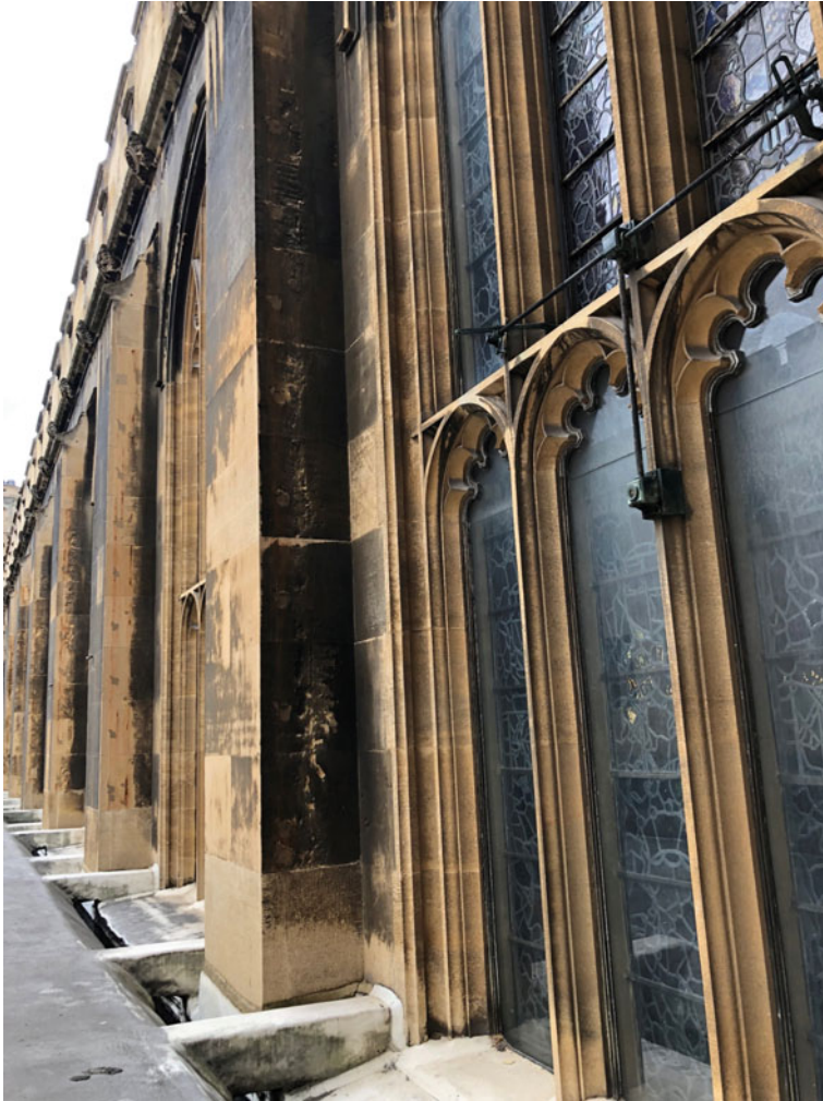
Fig. 13.12 Exterior of window in House of Lords, showing closing mechanism (Author's own photograph, 2019)
