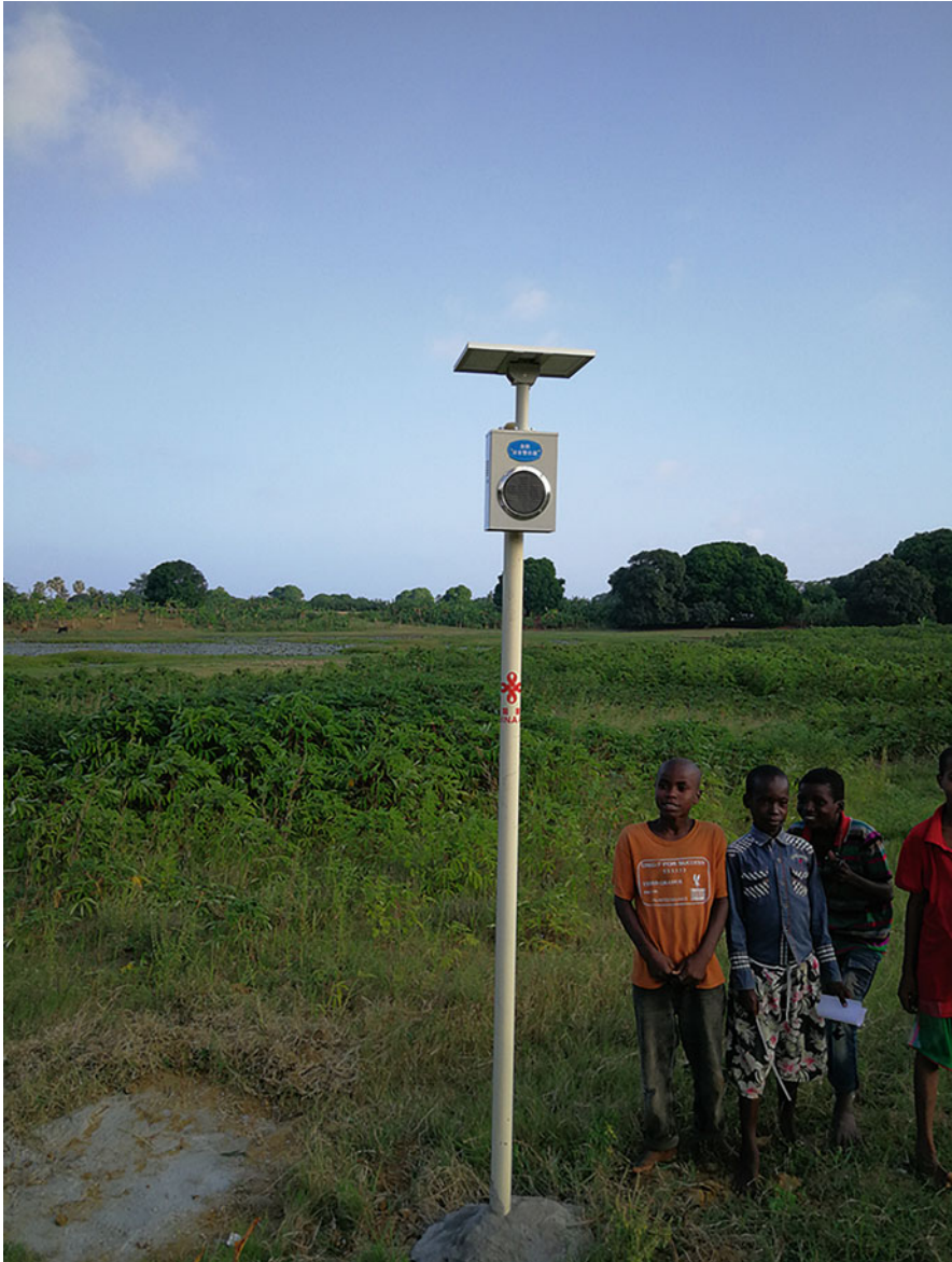
Fig. 11.8 A voice alarm machine in the risk area
