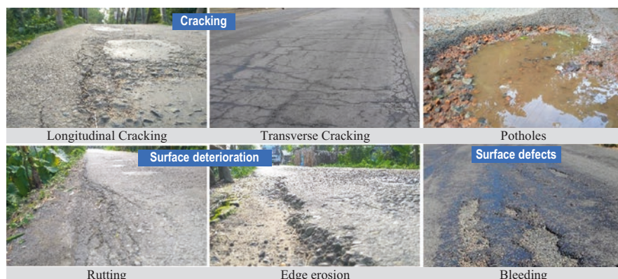
Fig. 2.8 Most frequent pavement damage types in the coastal area
