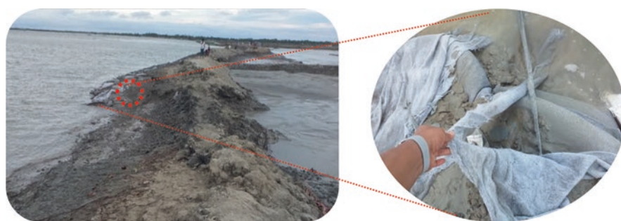
Fig. 2.6 Super cyclone Amphan washed out earthen embankments in Satkhira district (field visit: 10 June 2020)
