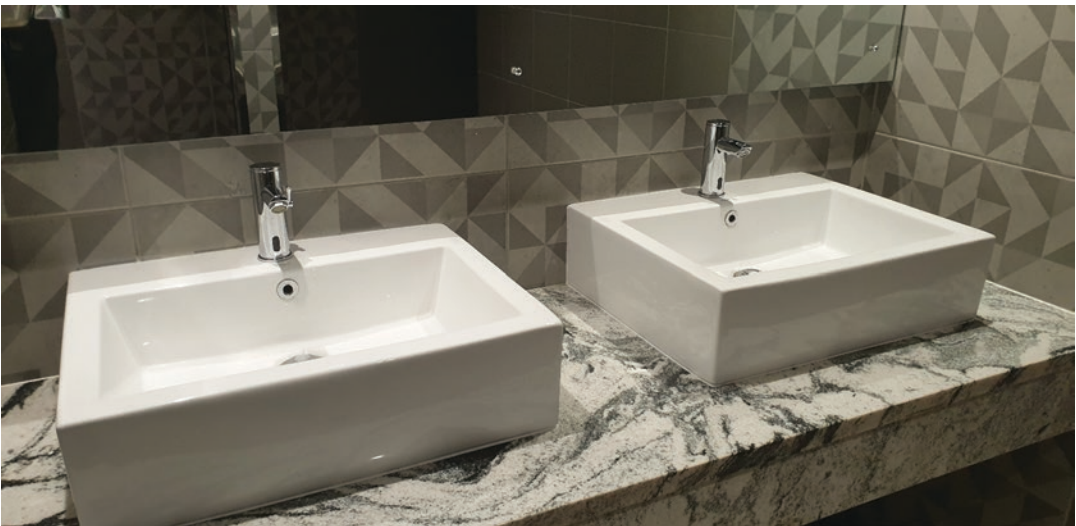
Fig. 13.7 Water-efficient installations in RR Maluleke Building. (Source: Authors)
