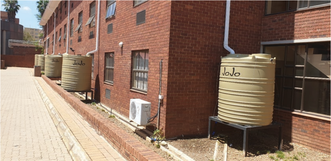
Fig. 13.6 Rainwater harvesting infrastructure at Sunnyside Campus. (Source: Authors)
