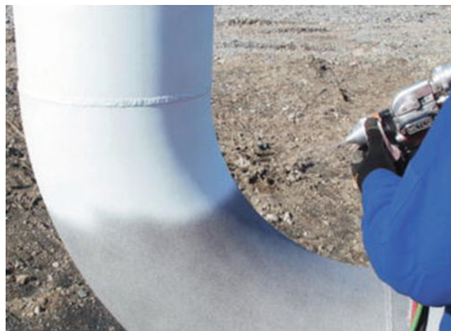
Fig. 19.20 Typical coating against corrosion sprayed on-site onto refinery pipe. (Courtesy of Oerlikon-Metco)
