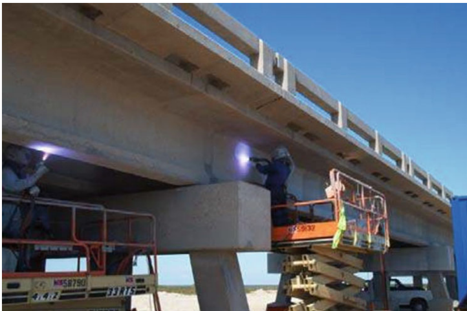
Fig. 11.61 Al/Zn/In wire arc spraying of concrete beams and caps of the San Luis Pass Bridge. http://www.metallisation.com/
