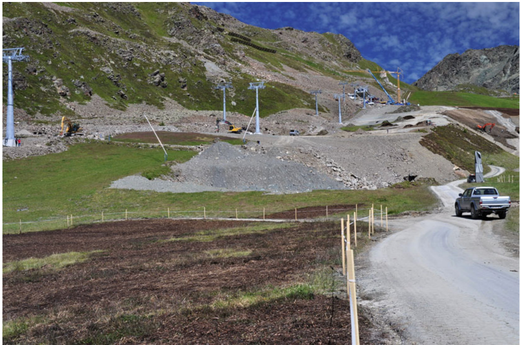
Fig. 1.56 Large tracts of land in the European Alps were reshaped in order to develop the ski industry as here above Ischgl, Austria, one of the top winter sport destinations in the Alps. (Photo © Udo Schickhoff, August 11, 2011)
