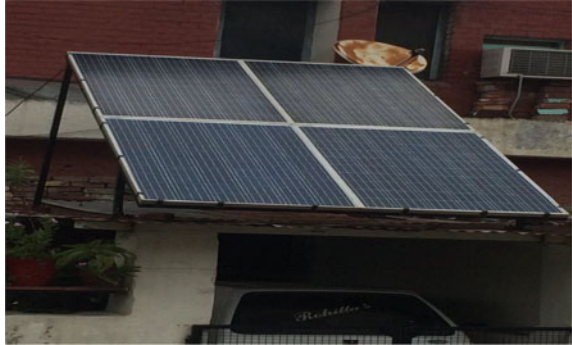
Fig. 4 4 Solar panels connected in parallel of 315 Watt each
