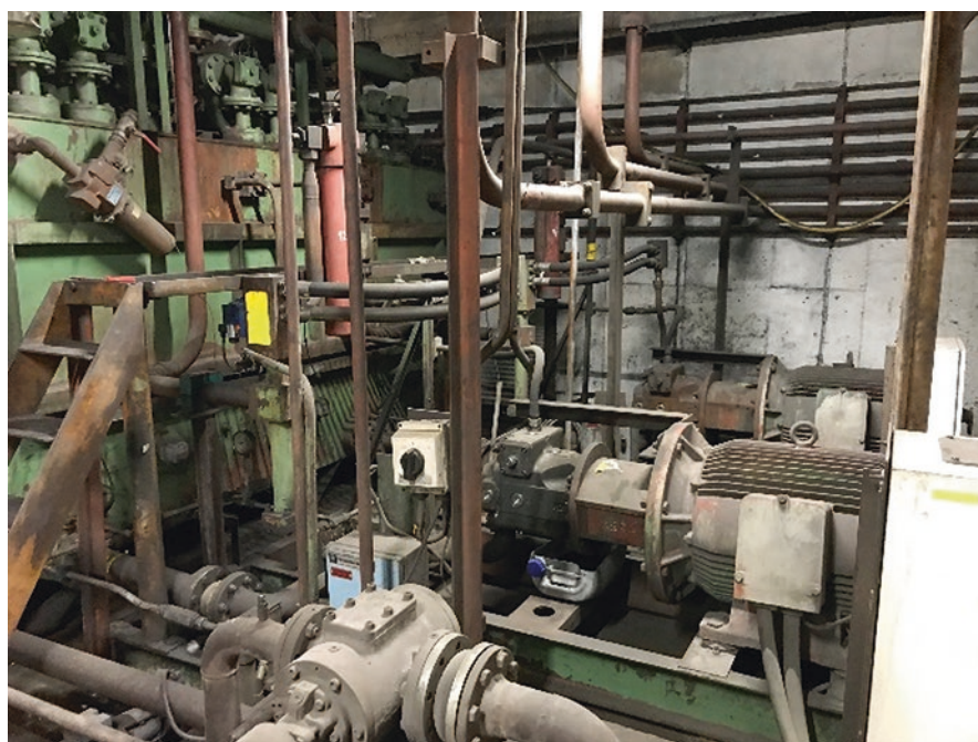
Fig. 8 Hydraulic pump 55 kW
