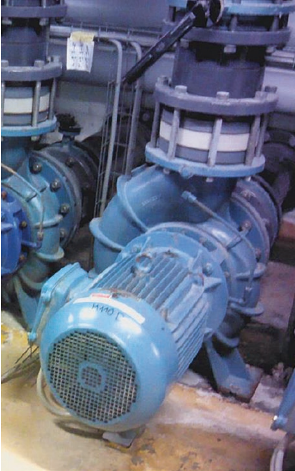
Fig. 5 13 kW lifting water pump installed in 1990, with a variable load regulated by a throttle (“Feinanalyse für Elektrische Antriebe ProAnalySys: Kurzbericht”, Electrosuisse, Fehraltorf (Switzerland), February 2018)
