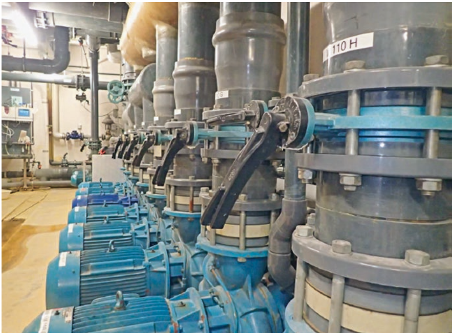
Fig. 9 The pumping system that was examined comprises seven pumps with a nominal power of 13 kW, six of which are in use for more than 4000 h a year. Regulation is mainly mechanical through the use of valves
