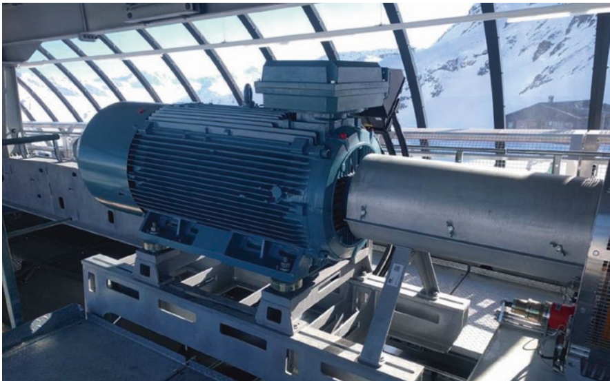
Fig. 3 Picture of the motor drive system of the cable railway
