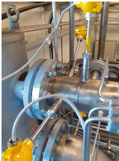
Fig. 4. Positioning of the temperature sensors at the turbine outlet duct
