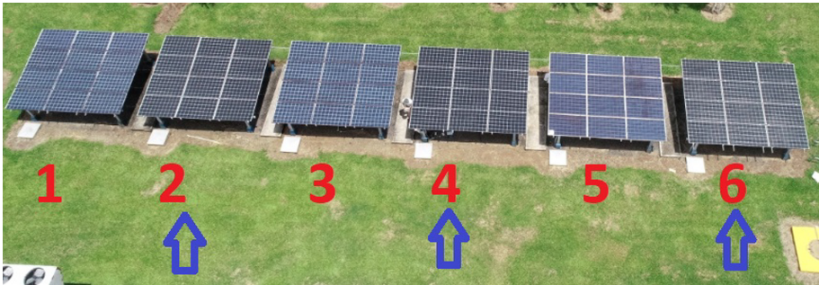
Fig. 3. Picture of the PV installation. Strings 2, 4 and 6 were used in this research.
