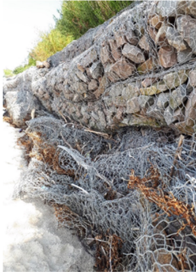
Fig. 4. 2019 The coastal line of the slope is preserved by a retaining wall: a) destruction of two rows of steps; b) an area where all elements of the gabion wall are almost completely destroyed.
