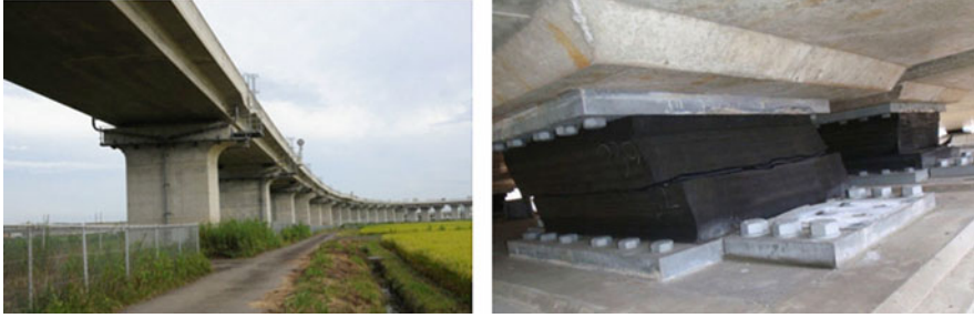
Fig. 5 Great East Japan Earthquake in 2011: bridge rubber bearings on the left and the horizontal crack is observed on the right [33]
