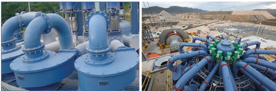
Fig. 1.6 A bank of classifying hydrocyclones (Courtesy: FLSmidth India Limited)
