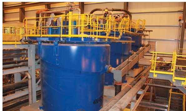
Fig. 1.14 A bank of flotation cells (Courtesy: Tenova India Private Limited)
