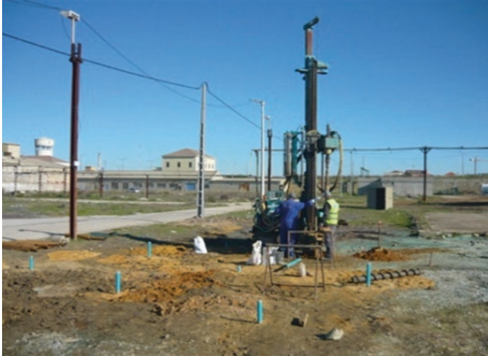
Fig. 11 Monitoring point's installation and general aspect of the Zone I field testing area
