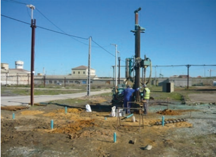
Fig. 11 Monitoring point's installation and general aspect of the Zone I field testing area
