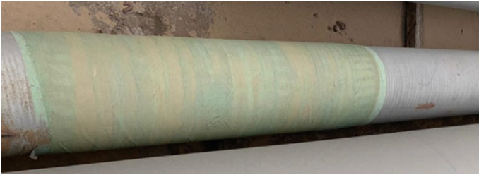
Fig. 2 This picture shows is a typical example of a defective pipe that was wrapped
