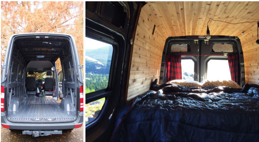
Fig. 6 Cargo van on day 1 (left) and interior of the van in 2016, after wall insulation and paneling, and storage and bed construction
