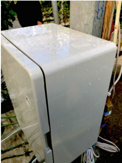
(a) Water condensation on the network equipment enclosure
