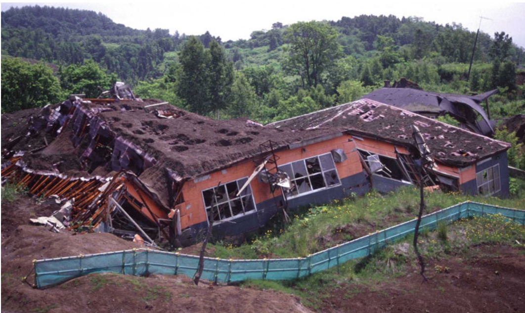
Fig. 1.25 Building damaged during the 2000 Usu (Japan) eruption. The damage is testified by the tilt of the building and the collapse of some of its parts, as well as by the impact of erupted ejecta on the ash-filled roof
