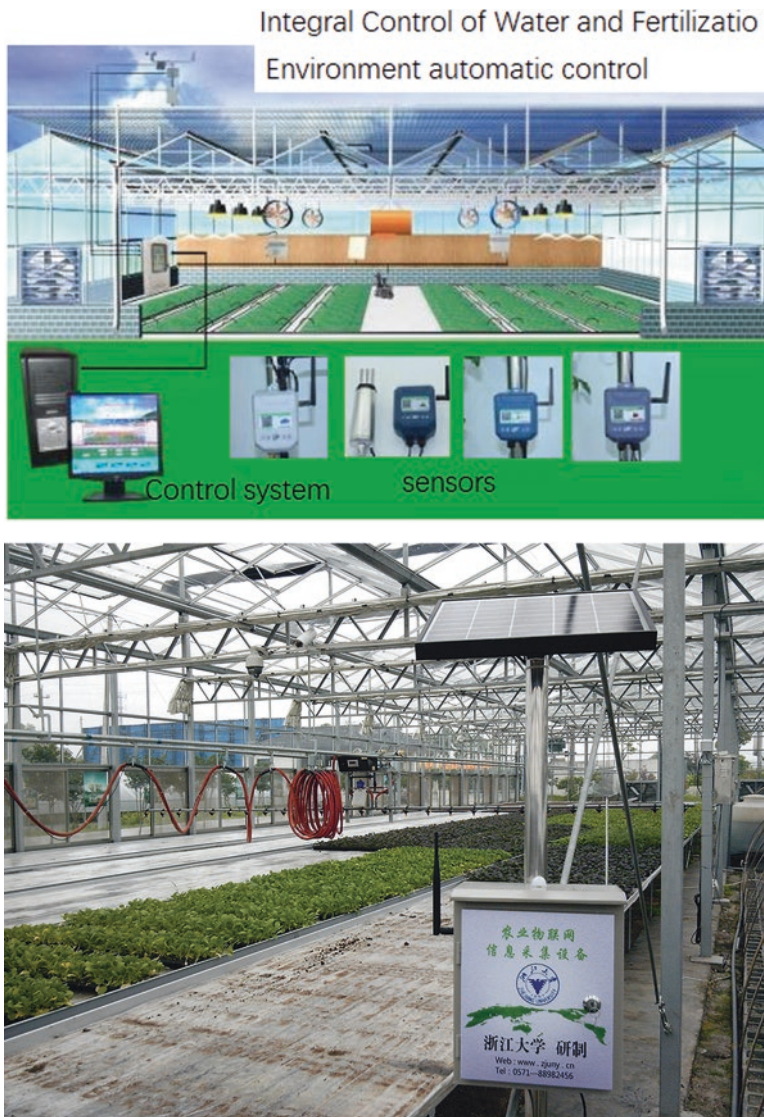
Fig. 11.9 Intelligent climate control systems
