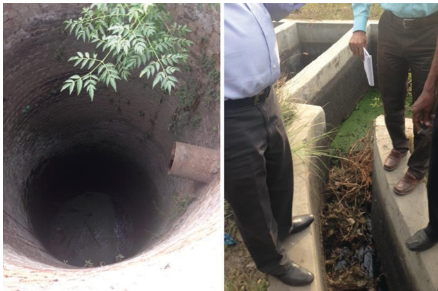
Fig. 10.3 A factory in Sheikhpura that has built unlined wells for the disposal of untreated effluent
