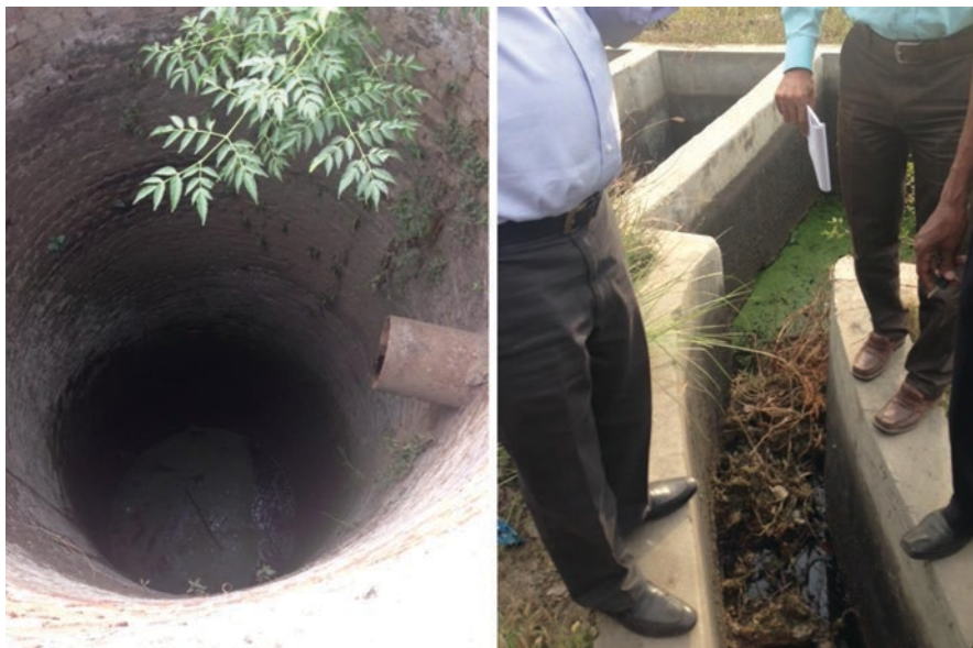
Fig. 10.3 A factory in Sheikhpura that has built unlined wells for the disposal of untreated effluent
