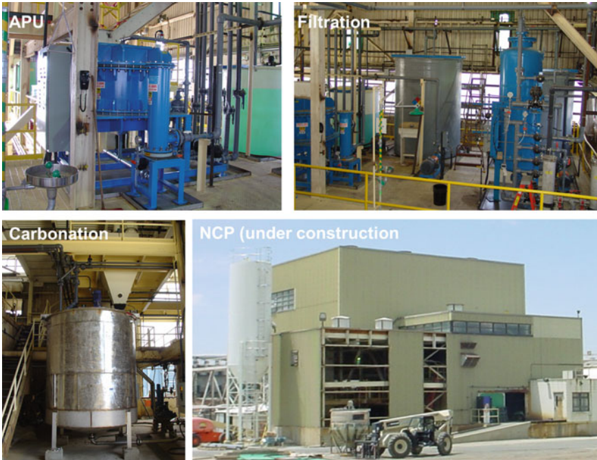
Fig. 5 Nickel carbonate plant—filtration-APU-purification-carbonation. (Color figure online)
