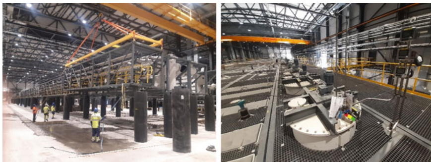
Fig. 7 Installation of modular SX units (left) and the view of multiple connected modules from above (right). (Color figure online)
