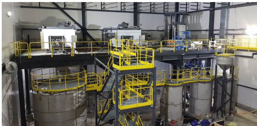
Fig. 4 Installation of filters and reactors in iron removal area. (Color figure online)
