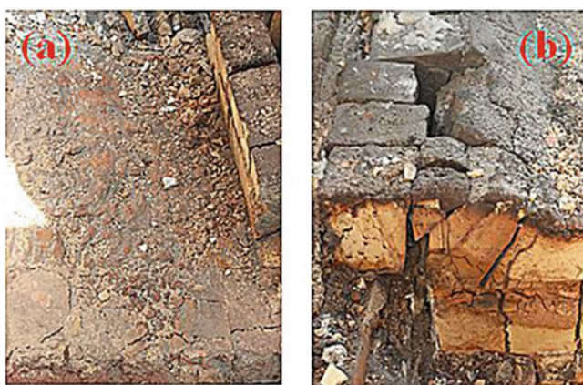
Fig. 4 Refractory material in the lower part of the bellows. (Color figure online)
