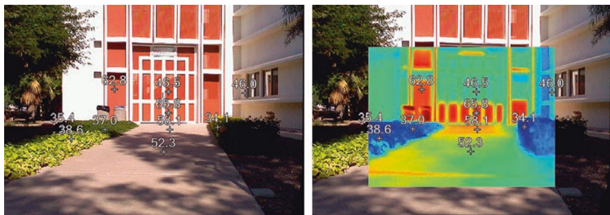
Fig. 8.11 Visible (left) and infrared photography (right) of case 1. False color scale is 30–70 °C
