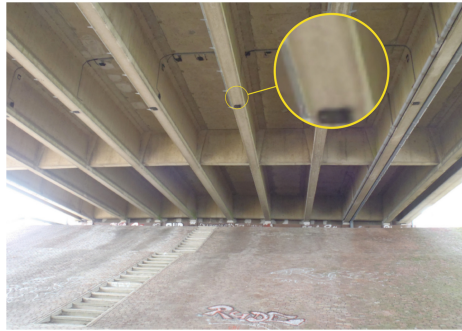
Fig. 2. Sensor locations at one of the girders of the bridge (from [16]). Sensors are either embedded or attached to the deck or girders.
