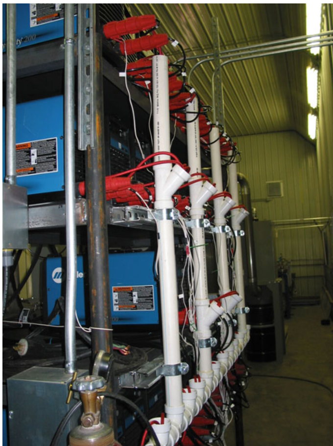
Fig. 10 The 26 electric arcing power supplies, 52 power and cooling water cables and cooling water discharge line. (Color figure online)
