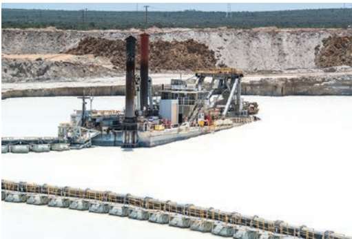
■ Fig. 2.20 Floating suction dredge. (Image courtesy of Tronox)
