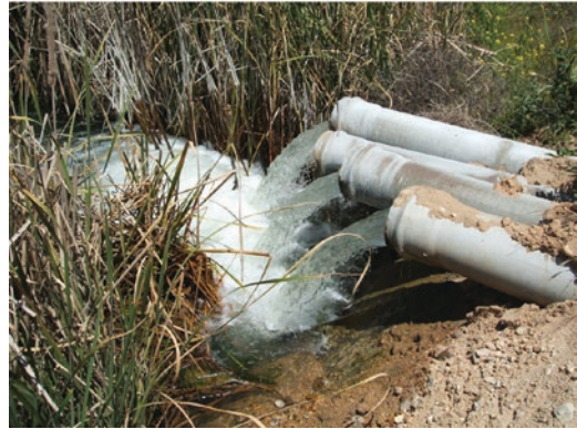
■ Fig. 2.18 Pumping water to draw down the water table. (Image courtesy of CEMEX)
