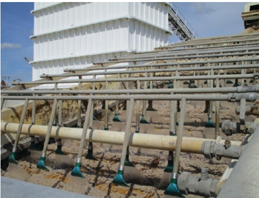
■ Fig. 2.34 Polyurethane nozzles for washing placed cross-sectionally to the material flow in a vibrating screen. (Image courtesy of SAMCA)
