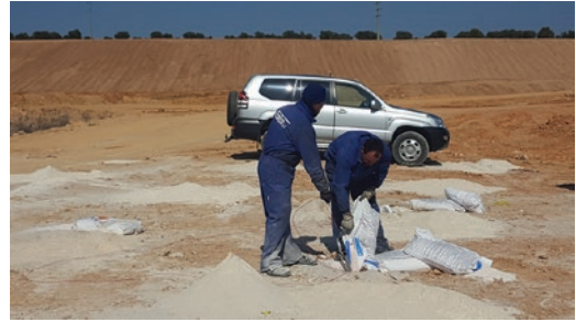
■ Fig. 2.21 Loading operation of ANFO nylon bags. (Image courtesy of Octavio de Lera)
