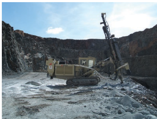
■ Fig. 2.8 Drilling in a crushed stone (andesite) quarry. (Image courtesy of Benito Arnó e Hijos, S.A.U)
