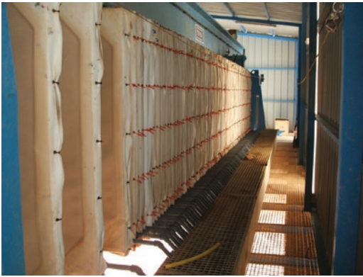
■ Fig. 2.30 Pressure filters for dewatering in an aggregate plant
