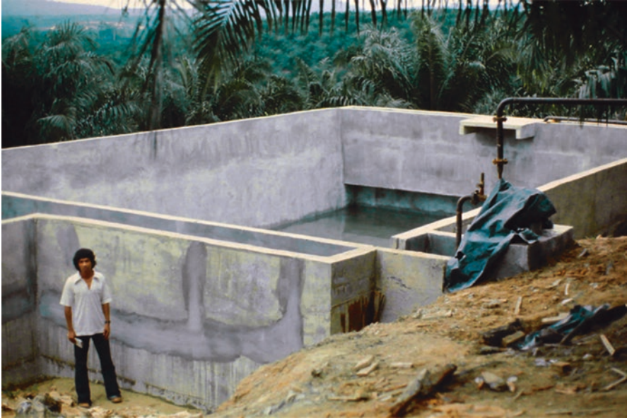
Fig. 13 Enlarged palm oil effluent holding tank in Pahang, Malaysia (1974)
