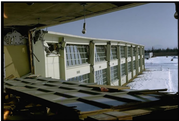
Fig. 1. Example of failure of non ductile reinforced concrete frames observed in the Alaska earthquake.
