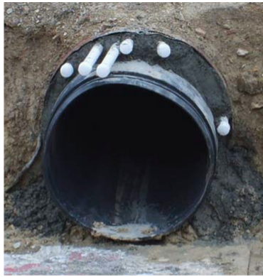
Fig. 1. Grouting the annular space between old pipe and lining pipe (Utah DOT)
