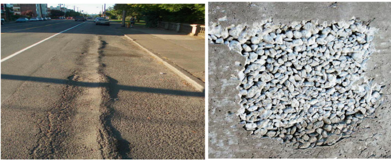
Fig. 1. (a) Rutting of asphalt and 1 (b) Honeycombing of hard pavement
