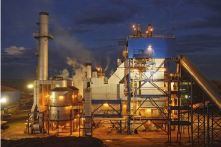
Fig. 20.4 A bioelectricity plant in Brazil. (Source: [17])
