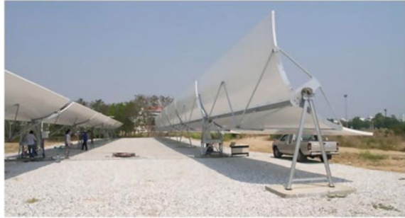
Fig. 9 Kanchanaburi concentrating solar thermal power parabolic trough plant in Thailand (Source [51])
