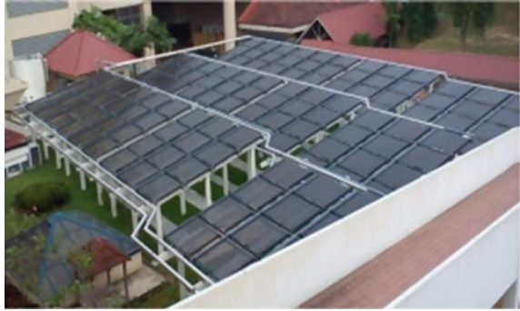
Fig. 7 Solar thermal system in Hospital Universiti Kebangsaan Malaysia (Source [48])
