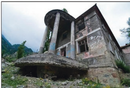
Community Centre. Deep scour under the stairs.
