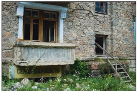
One of the houses of Belgian construction. The ground floor is completely covered with debris flow deposits. The store sign is on the ground level.
