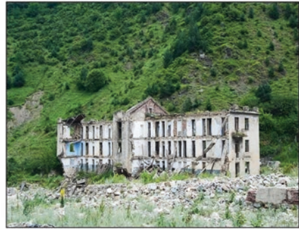
The building of the former office of Geological Exploration Crew (GEC). A third part of the building was destroyed and carried away by a mudflow.
