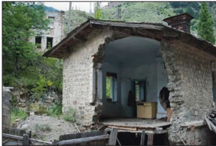
Ruined wall of a residential building.
