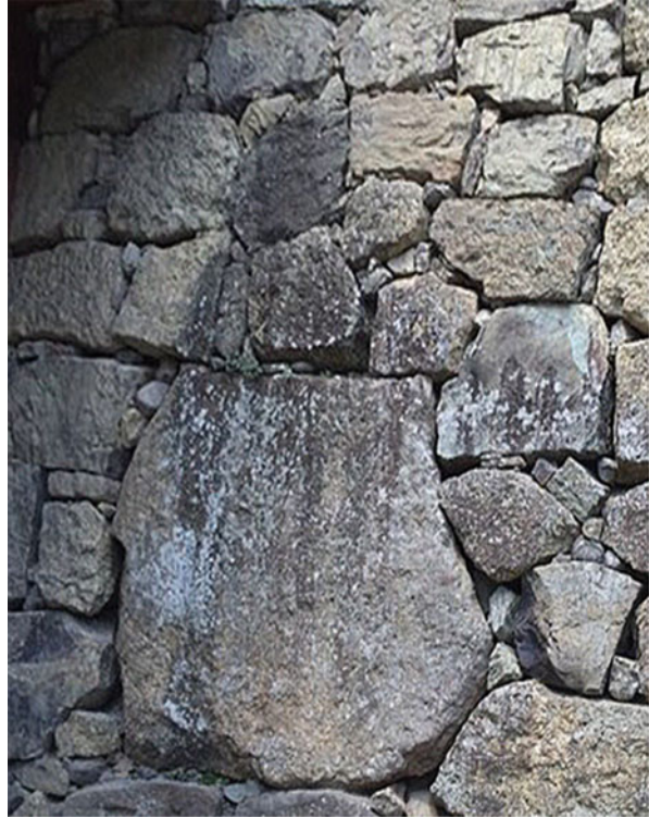
Fig. 25.4 Stone wall of the Ueda castle (Ueda, Nagano) consisting of various size of stones, including a large stone called Sanada stone
