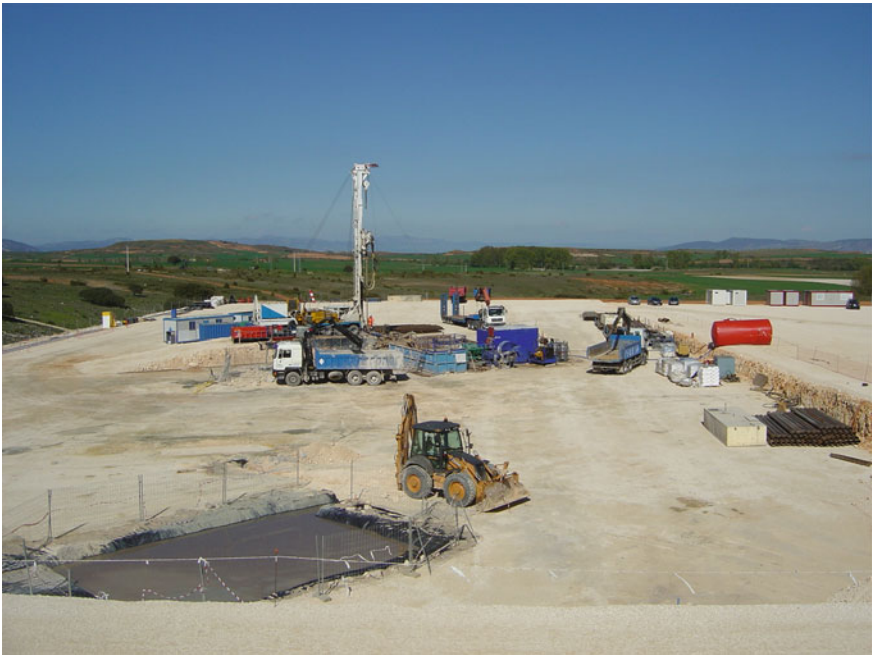
Fig. 4 Drilling on-site panoramic view with the rig and auxiliary equipment (Courtesy of CIUDEN)
