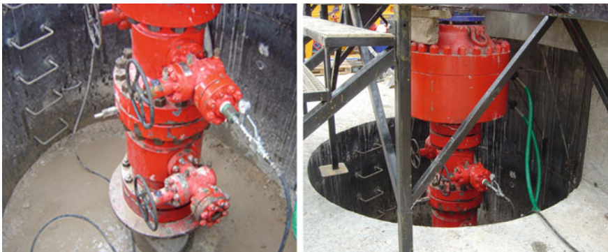
Fig. 6 Installation of BOP and spools during HI well drilling (Courtesy of CIUDEN)
