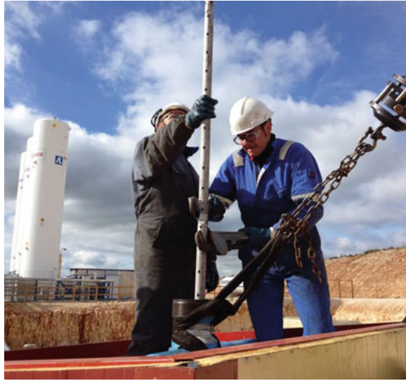
Fig. 13 Choke installation into the HI injection tubing
