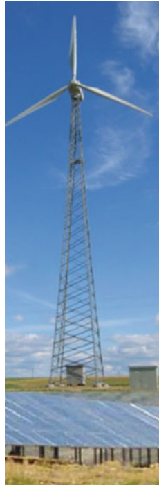
Fig. 21 Renewable power plant created in Silifke-Turkey
