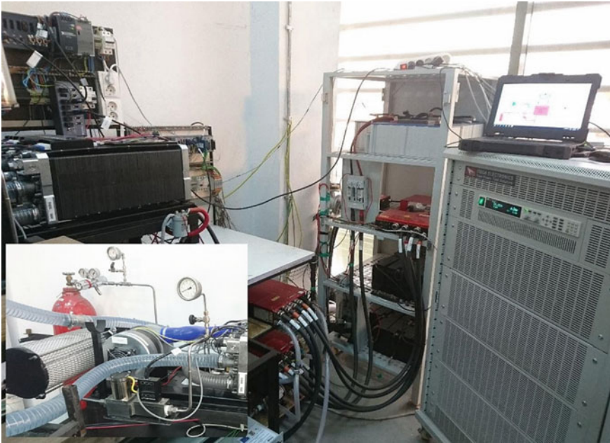
Fig. 17 Experimental installation for FCHEV testing
