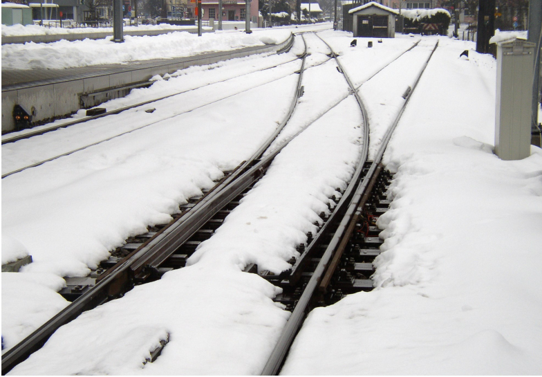
Fig. 1. Gas heating keeping a railroad switch free from snow and ice (Di Fabian Grunder (FabiBerg) – Opera propria, CC BY-SA 3.0, https://commons.wikimedia.org/w/index.php?curid=641923 )
