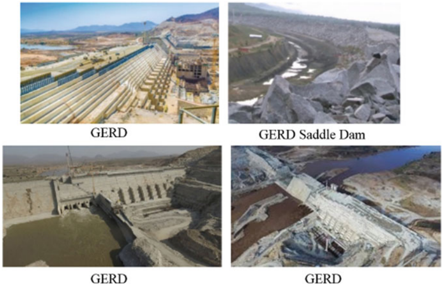
Fig. 2 Progress of construction in the GERD and the auxiliary Saddle Dam as of 2017
