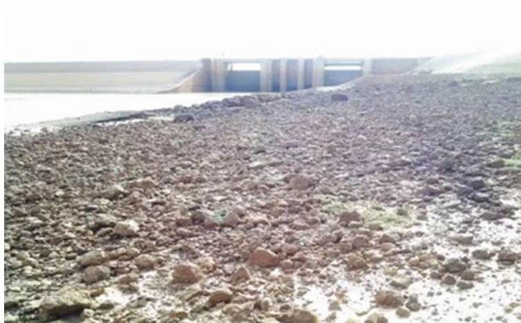
Plate 4 Sand Dome presence in Goronyo Dam
