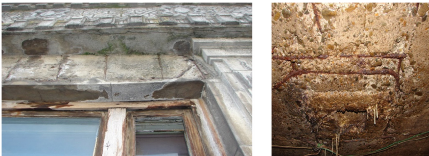
Fig. 8. Plaster efflorescence and exfoliation followed by steel reinforcement corrosion
