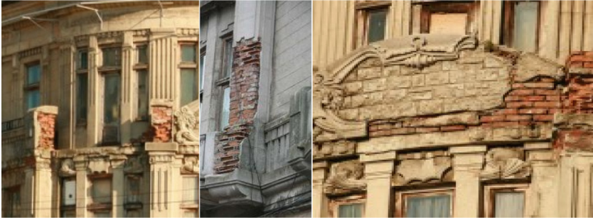
Fig. 9. The severe damage of the masonry elements and of the architectural finishes [16]
