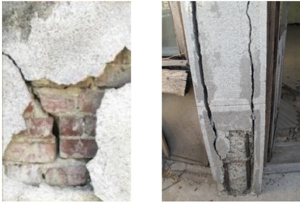
Fig. 6. Cracks developed in the concrete cover and in the elements of the super-structure [16]
