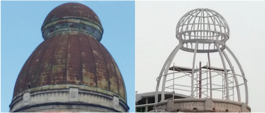
Fig. 11. a) The dome metal covering badly affected by the environmental conditions [16]; b) current rehabilitation stage
