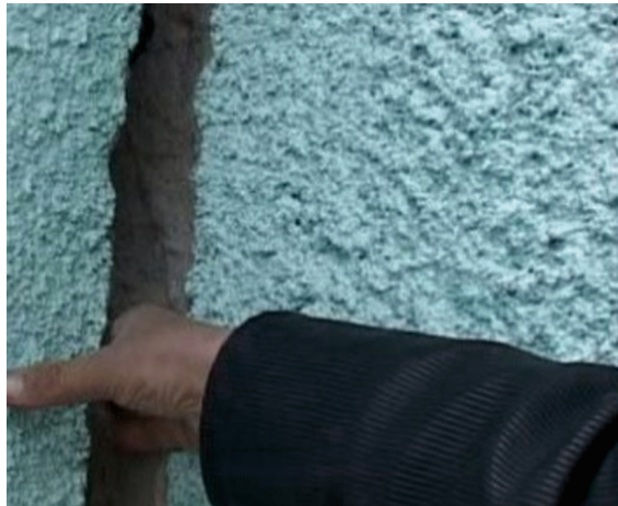
Fig. 16. Cracks in the walls, Pârcovaci village, 1996
