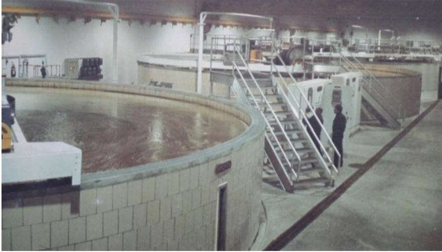
Fig. 8.5 The Heart of the Pittsfield WTP is 6 DAF-filtration clarifiers (DAFF, Krofta Sandfloat SAF49), each being 49-ft in diameter, 6-ft in depth, treating 6.25 MGD
