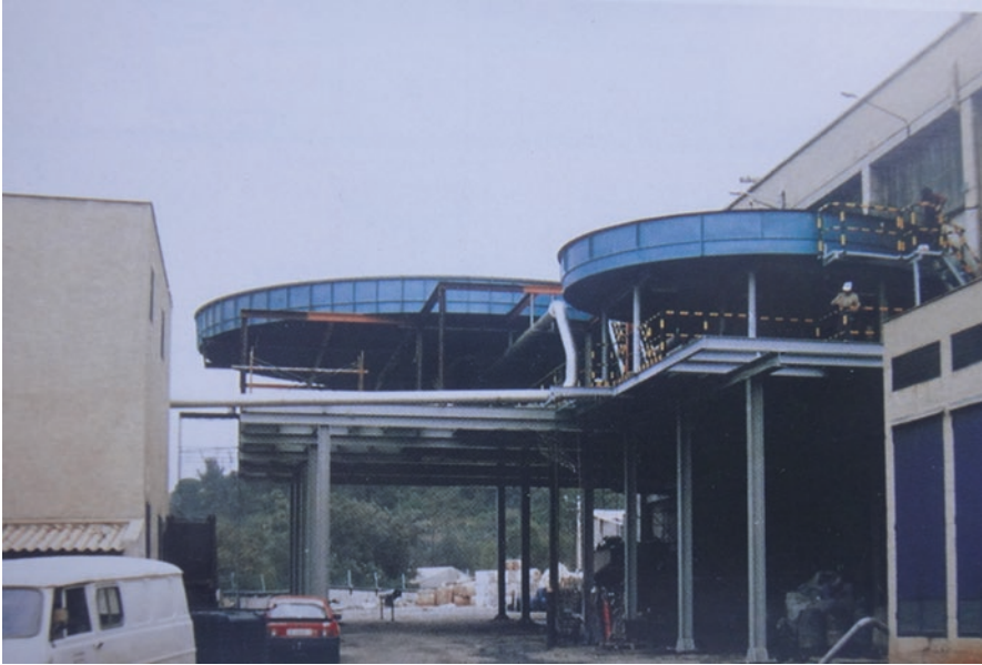
Fig. 6.17 Two elevated light weight shallow circular dissolved air flotation clarifiers with zero footprint [162]
