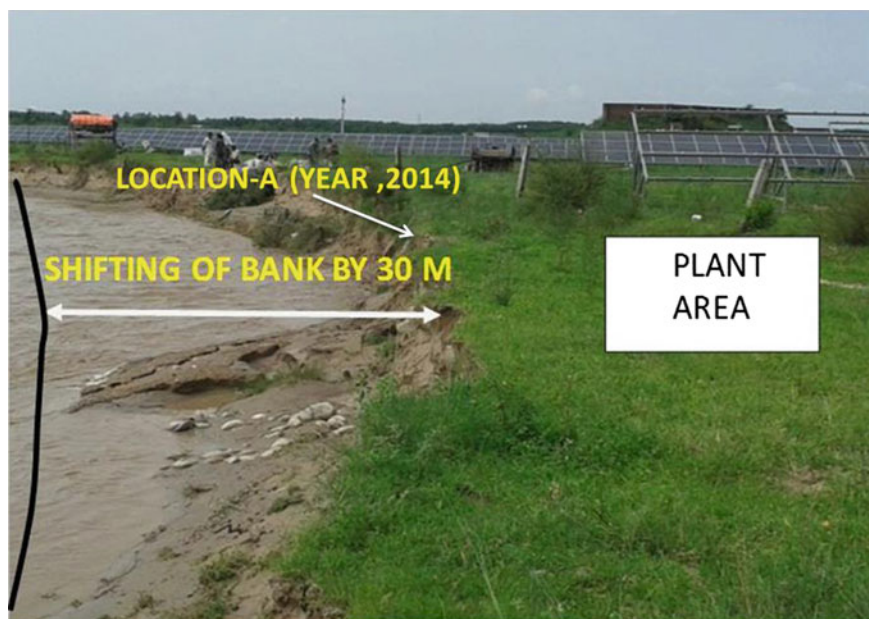
Fig. 5 Scouring of the left bank during monsoon season, 2014 in Solani River. Left bank in front of the plant got shifted by about 30 m by initial monsoon flood of the year 2014 (Fig. 4)
