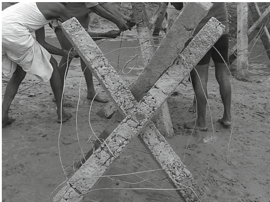
Fig. 7 RCC Jack-Jetty of 1.5 m length, 0.1 m width, and 0.1 m thickness meshed with 4 mm galvanized iron wire
